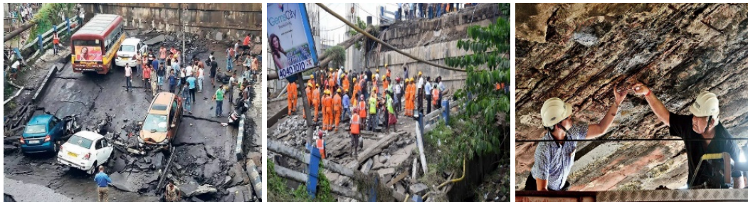
Fig. 1. (a), (b) Catastrophic failure of bridges; (c) distress in bridge deck.
